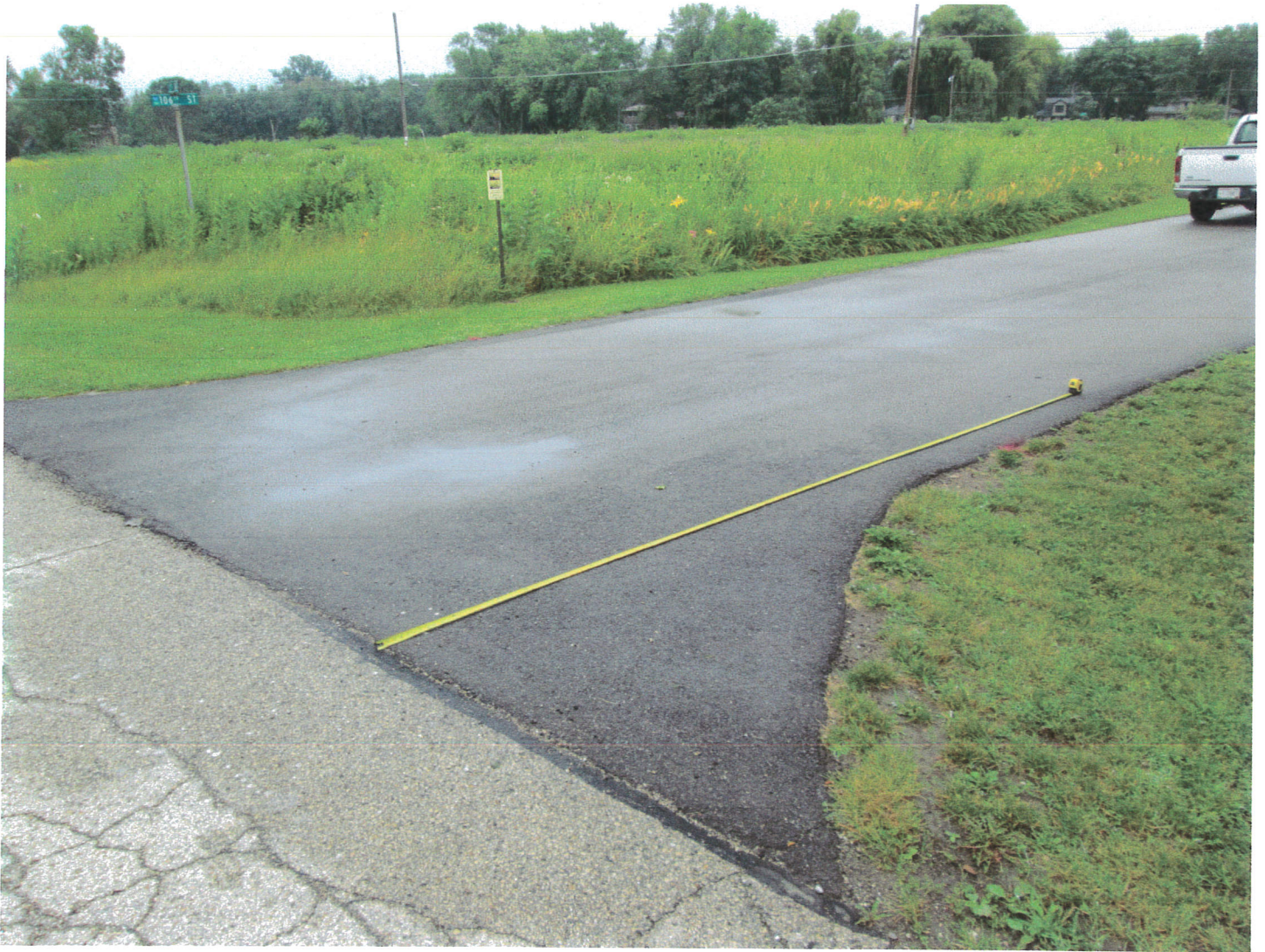
Driveway with paint markings for paver / asphalt boundaries.
